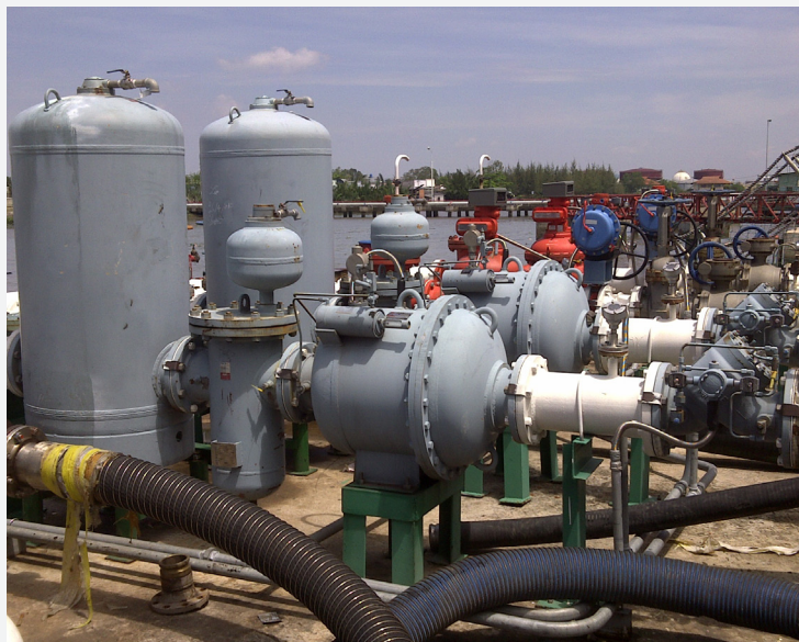
BiRotor Meters and Control Valves [Ship Loading/Unloading]
