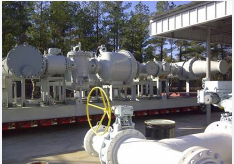
Pipeline Metering Skid on a Brodie calibration stand
