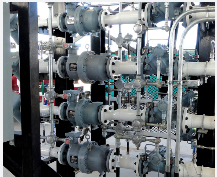
BiRotor Plus Meters and Control Valves [Truck Loading]
