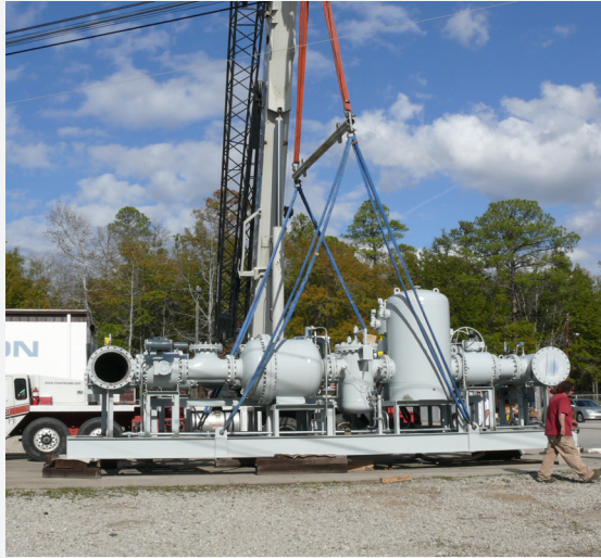
Pipeline Metering System
